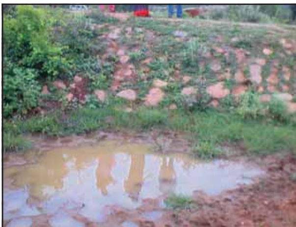
A failed water harvesting structure due to lack of support mechanism at village level- Chintapatla, near Ibrahimpatnam
